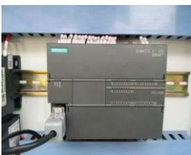
SIEMENS PLC Control System
