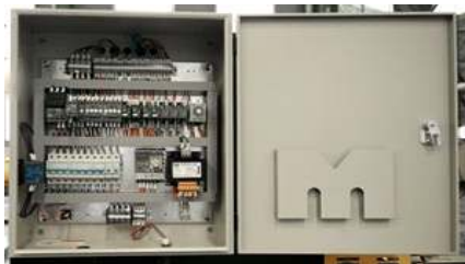
France Schneider Electric Controls
