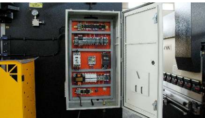
France Schneider Electric Controls
