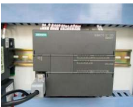
SIEMENS PLC Control System
